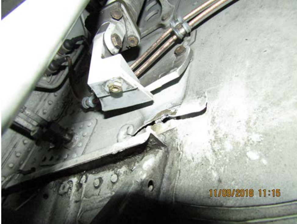
Figure 2: Broken bracket viewed from below shows damage to fitting attachment
