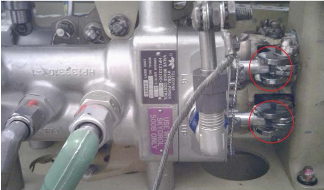
Fig 4: Challenger 601 brake valve installation showing plungers contacting brake levers.
