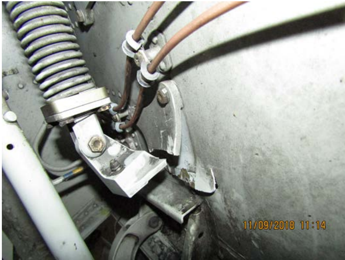
Figure 1: Broken bracket viewed from front
