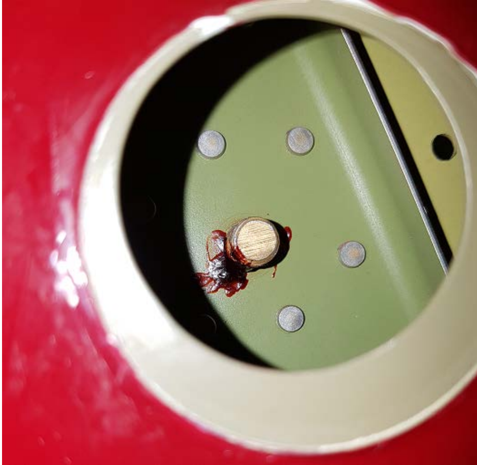
Pic #2 Missing nut and washer
