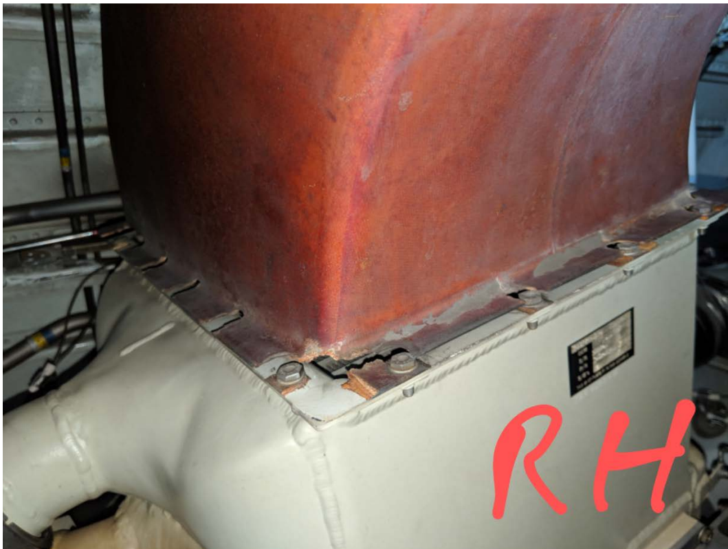
Fig 4: RH duct inboard and front showing separation from heat exchanger
