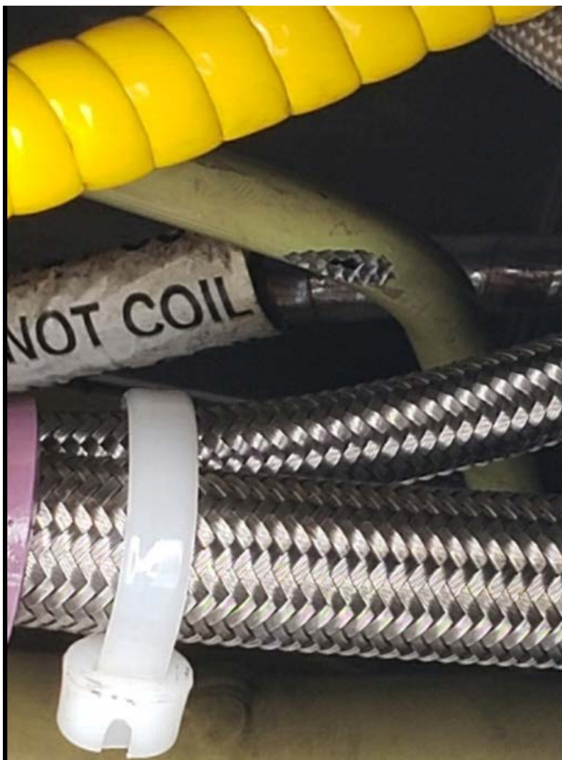
Chafed oil fill line
