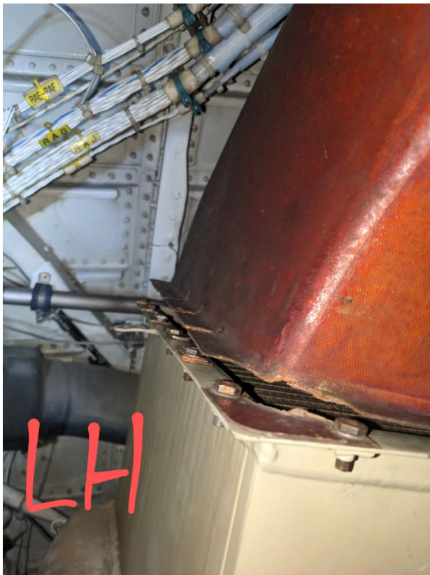
Fig 1: Left-hand (LH) duct aft and outboard showing separation from heat exchanger
