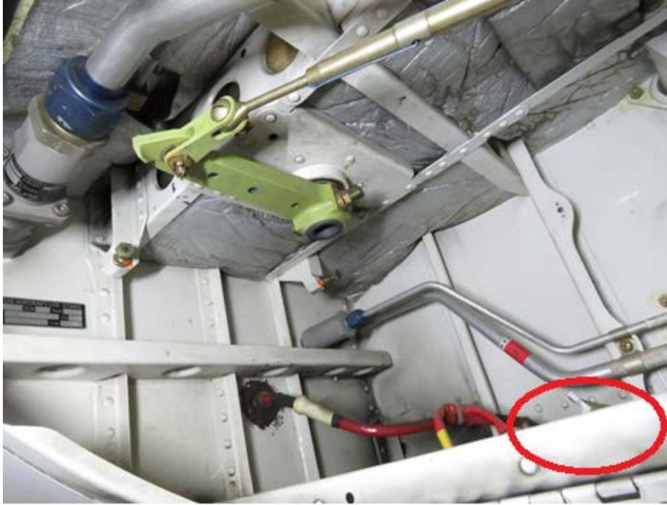
Pic. 1 Bellcrank assembly as found by maintenance prior to removal. Broken piece of bellcrank (circled) found on floor of cavity.
